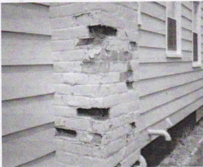
Michigan attorney E. Powell Miller says homeowners should have been warned of possible damage like this from orphaned water heaters.
