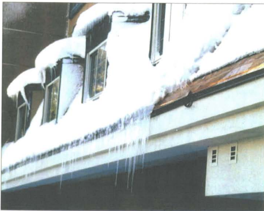
Heated eaves are one cure for ice dams. Warmed by electric cables, the copper eave in the foreground prevents ice dams that can cause leaks in the roof. The icicle-encrusted eaves in the background don't have heated metal eaves.
