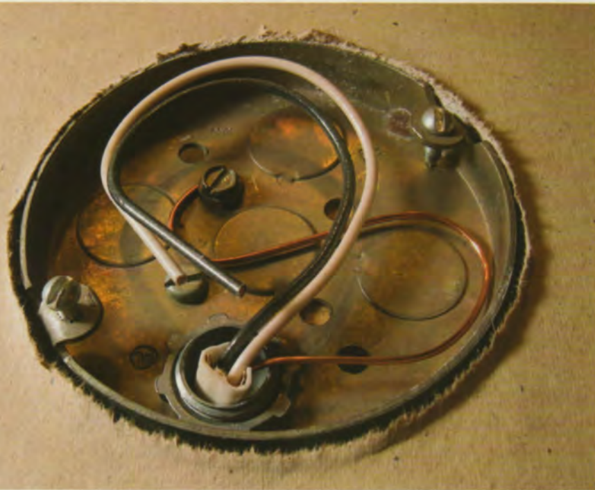
Photo 1. This ceiling pan, with a volume of 6 cu in. and no required fill adjustments for an internal cable clamp, can just accommodate a single 14-2 AWG Type NM cable, or a 14, 12, or 10-2 AWG Type AC cable.
