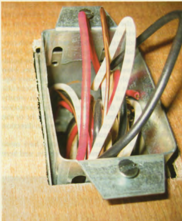
Photo 3. This is one example of an extension for recessed device boxes. The device has been omitted to give a better view of the ring. These extensions are now available for round outlet boxes, and in nonmetallic configurations.
