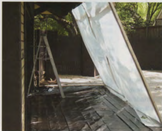
To contain paint chips and dust in windy conditions or when the work site is closer than 10 feet to another building or property line, the EPA now requires vertical containment. This can be as simple as propping a plastic-covered 2x4 frame against the eaves.
