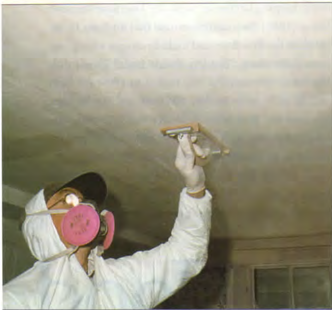
Sandable Durabond eases the final touchup, even over plaster. A Tyvek suit and charcoal mask are musts when sanding old buildings.
