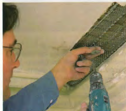
Expanded metal mesh is the modern lath common since the 1920s and widely used for large repairs. Here, a piece is cut to the patch shape and screwed right over the old wood lath to improve anchoring for the plaster scratch coat.
