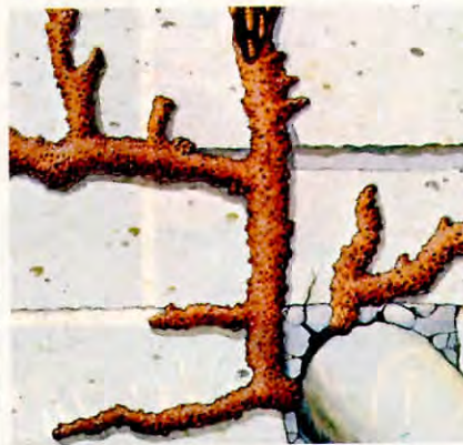
Termites may build a network of tubes along foundation walls to shelter themselves from light and air as they travel from the soil up to the food source—the wooden parts of a building.
