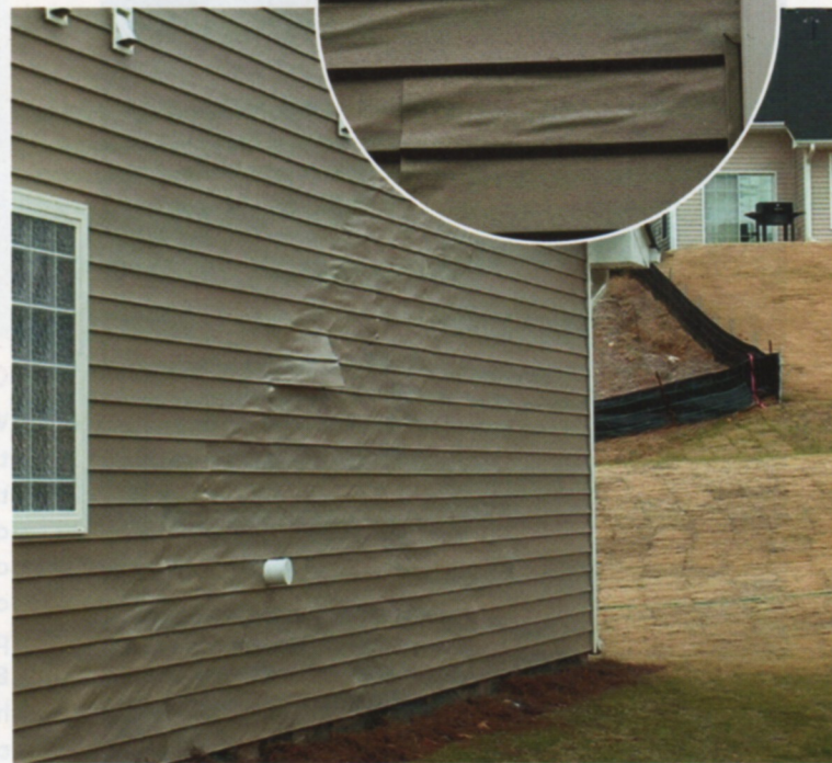
Unforeseen siding effects. As modern windows get better at reflecting the sun’s energy, homeowners with vinyl siding are paying the price. The melted siding shown here was caused by sunlight reflected from windows on the house next door. The diagonal warping pattern shows the sun’s path as it travels across the sky.
