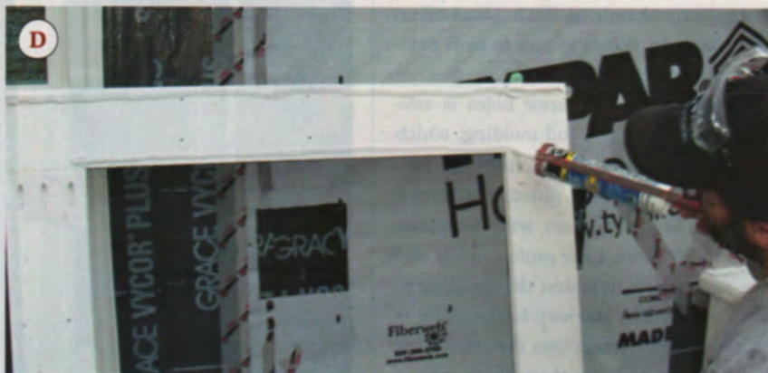
Figure 10. The backs of the prepared sill and casings are drilled for pocket screws (A). Facing surfaces are then coated with PVC cement and temporarily clamped together while the screws are driven (B). Next, the completed trim assembly is drilled for the deck screws that will fasten it to the framing, and caulked on the back before being lifted into place (C, D).
